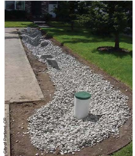
SUBSURFACE INFILTRATION COLLECTING DRAINAGE FROM AN IMPERVIOUS AREA
