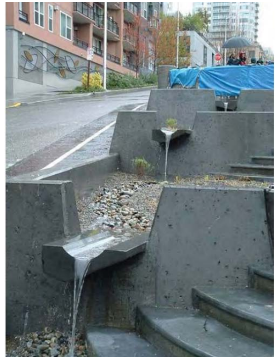
RIVER ROCK SWALE
