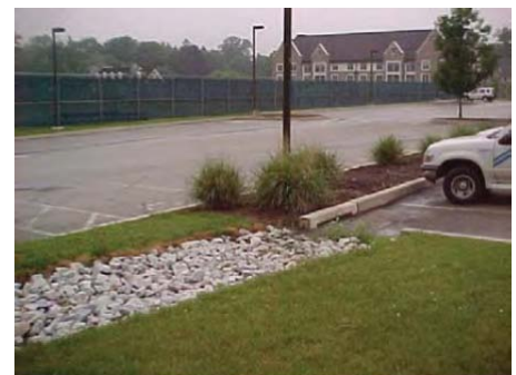
FILTER STRIP PROVIDING PRETREATMENT FROM A PARKING LOT TO A BIORETENTION SYSTEM
