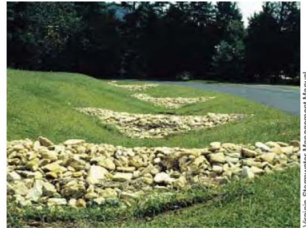
CHECK DAMS: NOTE CHANNEL STORAGE CAPACITY CREATED BY CHECK DAMS. NOTCHED CENTER ALLOWS SAFE OVERFLOW WITHOUT SCOUR AROUND SIDES
